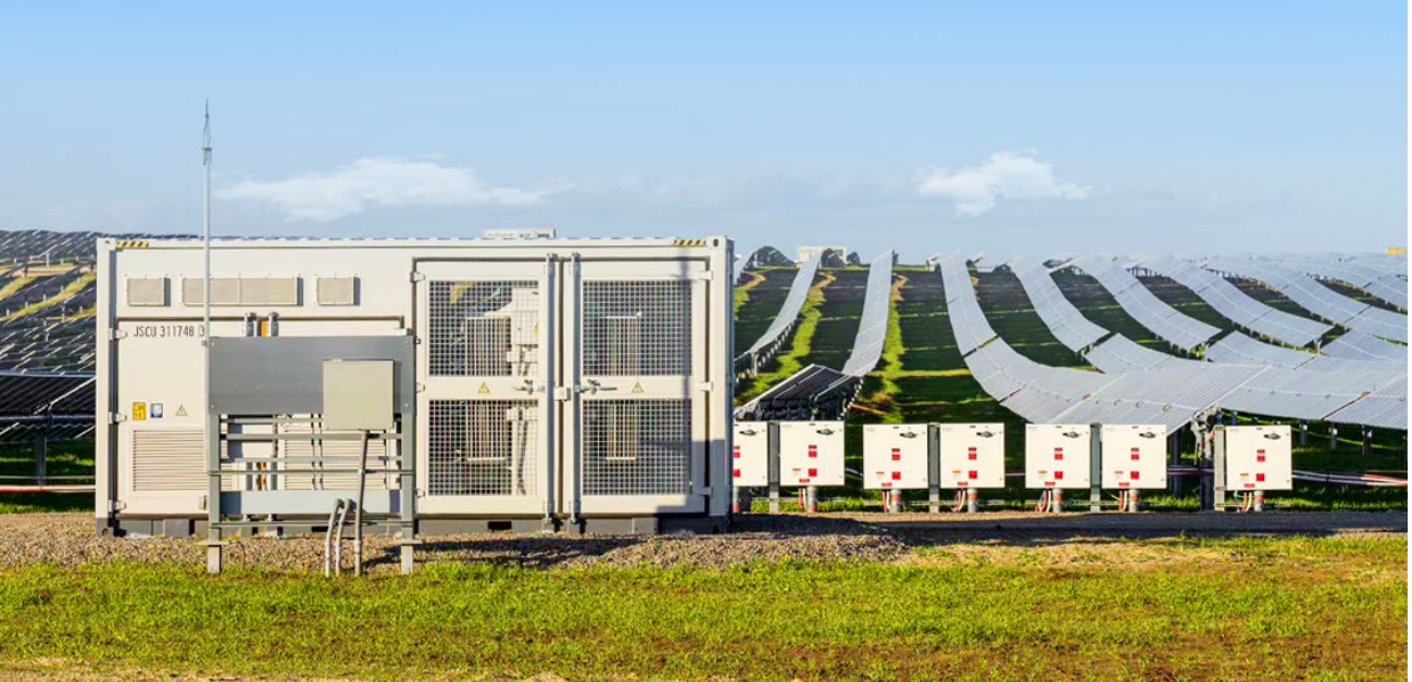
Fig-5: 200MW plant using central inverter + bifacial modules + tracker in California, USA
