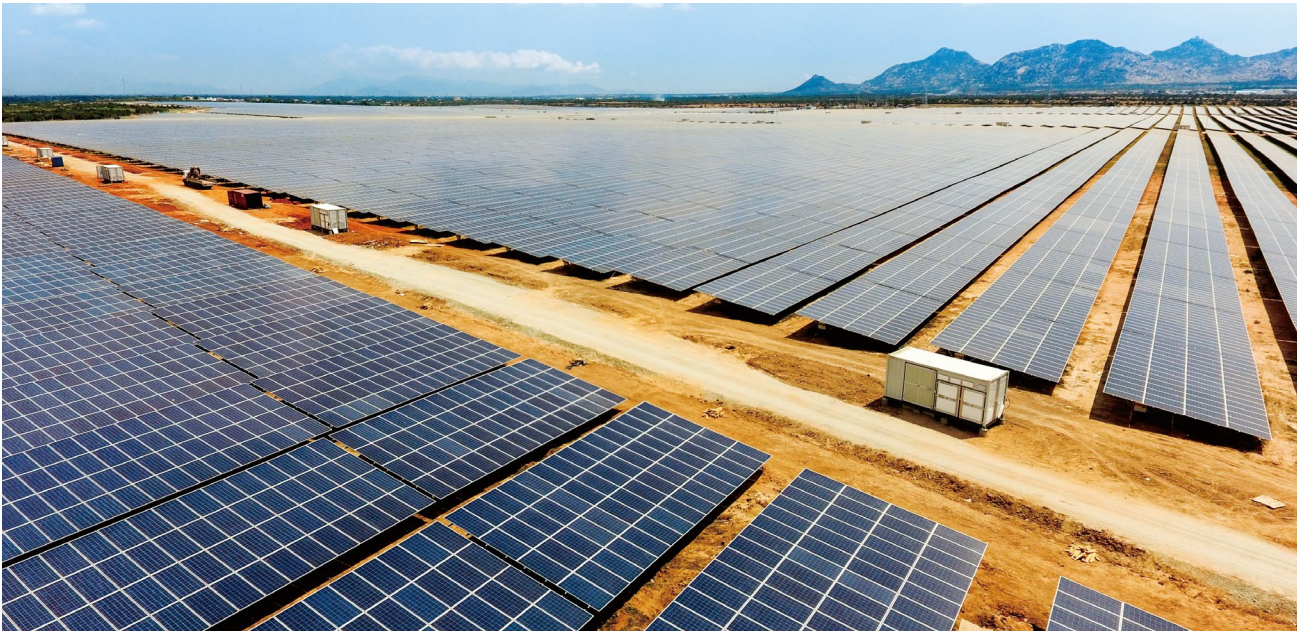
Fig-8: The utility-scale PV plant in Vietnam using Sungrow central inverter solution
